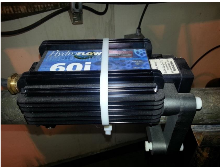
HydroFLOW 60i placed on water line feeding the RO system
